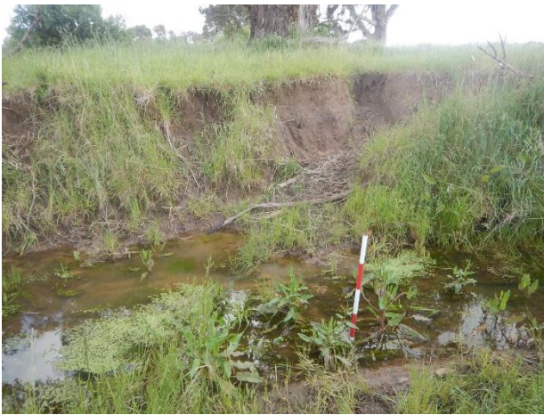
Photograph 5 Owens Creek showing erosion of banks (D.Carpenter, 16/11/2021, facing west)
