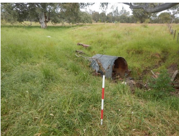
Photograph 7 Building material dumping in drainage channel in north-west corner of SU1 (D.Carpenter, 16/11/2021, facing west)
