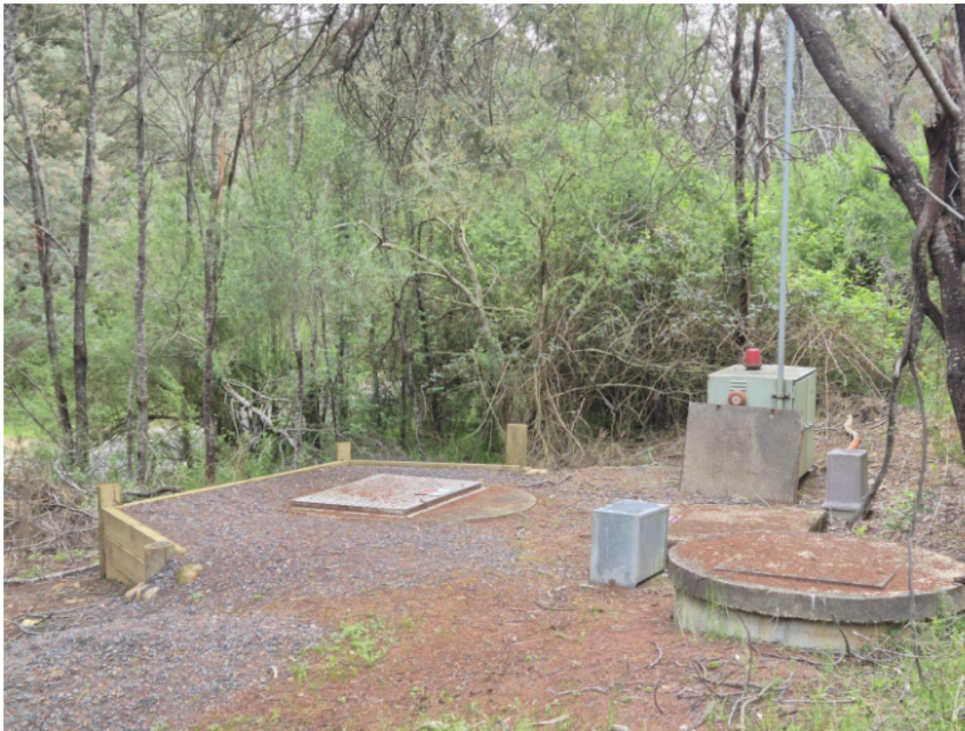
Image 1: Goulburn Valley Water Sewer Pump Station 01
