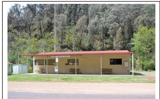
Works undertaken at Gaffney's Creek – 2 x 22,000 litre water tanks adjacent to the Community Hall.
